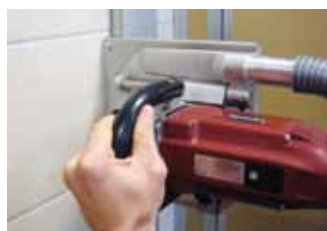
Cut into the tiled wall
