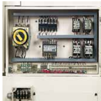
CLEAN, SIMPLE DESIGN AND WELL MARKED ELECTRICS MAKE MAINTENANCE ON THESE LATHES EASY!
